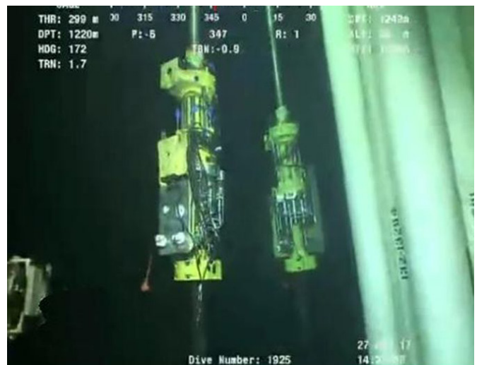
06 // CSS MORGRIP® 4 " Remote Connectors installed
